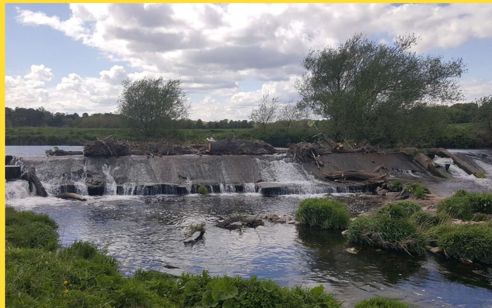
Knowes Weir with debris and no working fishway, River Tyne, Scotland, UK © Forth Rivers Trust
